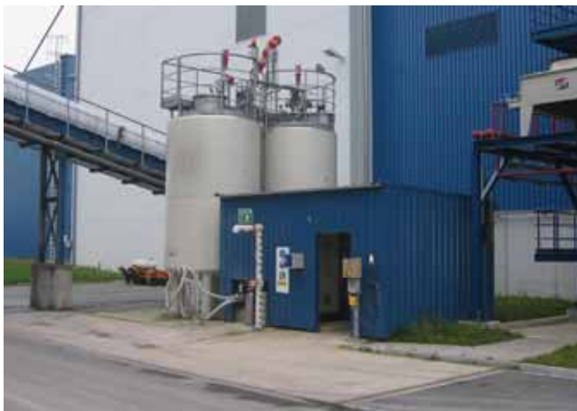
Figure 14: Storage Tank for Ammonia Water with Pumping Station
