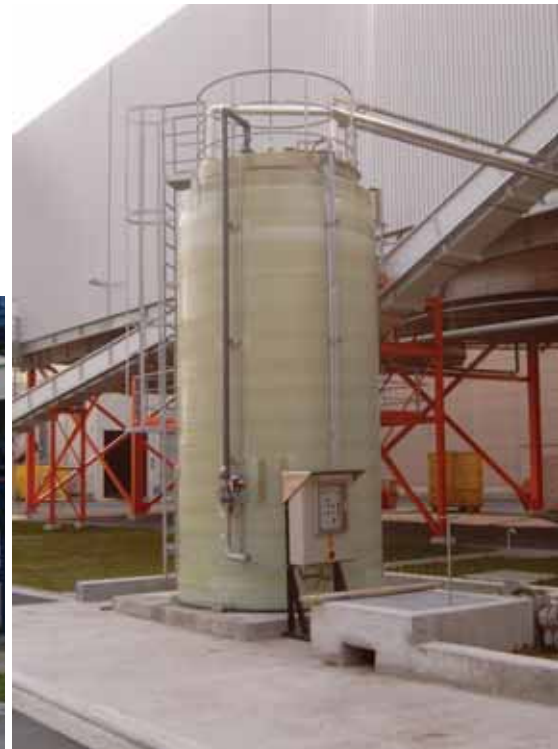
Figure 15: Storage Tank for Urea Solution
